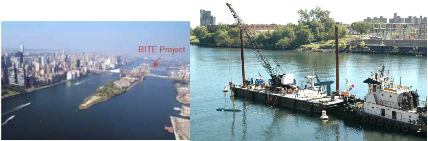
Figure 66 Location of the RITE project with the turbine being installed in September 2008 [91, 92]
