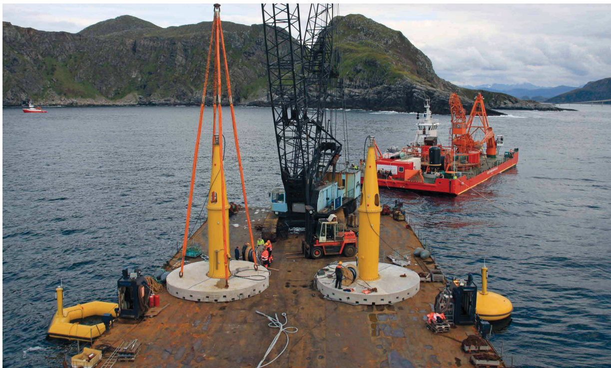
Figure 30 The two WECs being installed at the Runde test site, showing the buoys(in the water) together with the linear generator and gravity foundation (on the barge) [40].
