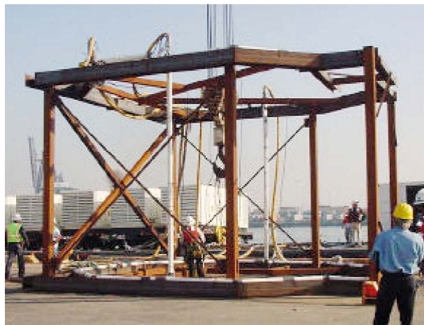
Fig. 3-15. Two-ring bubble curtain system. The white containers in the background are compressors (Reyff 2003).
