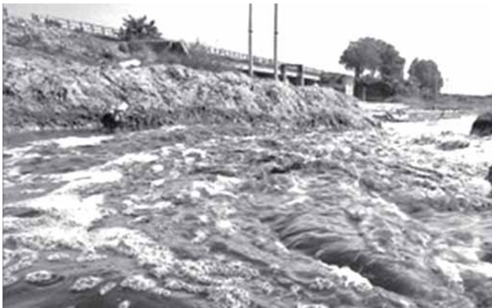
Figure 7 : Sea wall erosion
