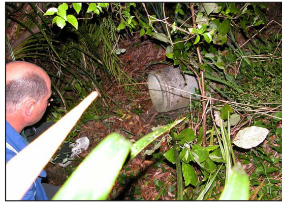
Figure 8. Main causes of malfunctioning amphibian mitigation measures II.: construction problems (tunnel entrance over the ground), besides the fence is lacking (near Auckland, New Zealand). (Photo courtesy: Dr. Phil J. Bishop)
